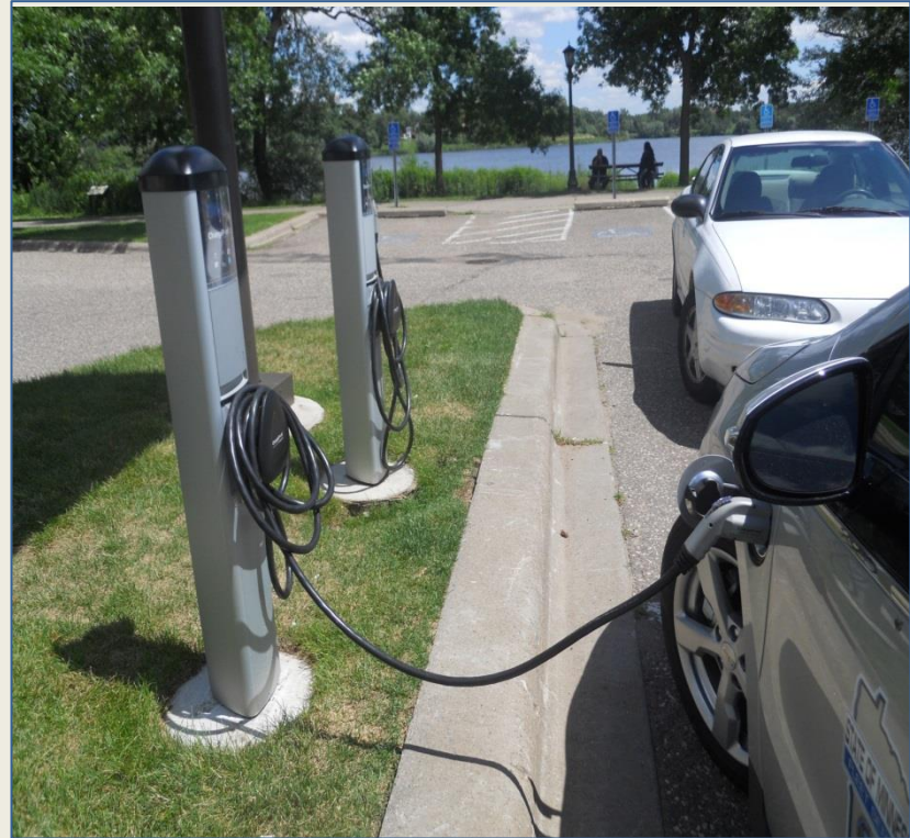
Charging with Solar Electricity Como Park in Saint Paul
